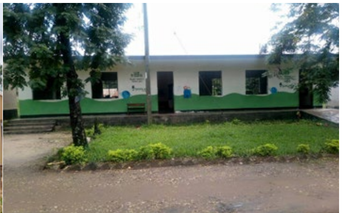
Kiloka Primary School – Morogoro, Two classes and desks. Handover planned to be in May 2024
